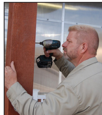
Hyrum Thompson, the founder of Western Timber Frame™ installing a timber frame pergola.
